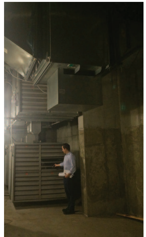
Commissioning Engineer Philip Karnicki illustrating the change in airflow through a set of fatigued return air dampers when forced open.
